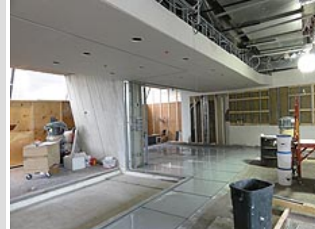
Floor, wall and ceiling work are under way in the new remote operations center. Photo: Steve Dixon, FESS
